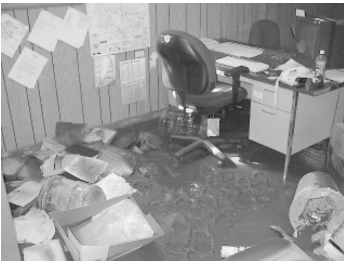
Recent Flood Damage to Welch Parole Office.
